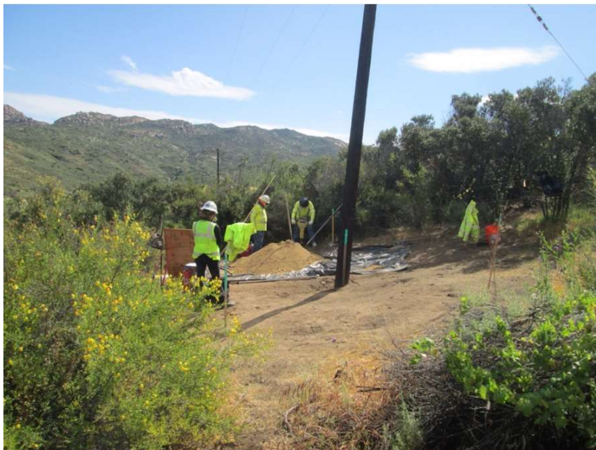
Photo 2: During pole anchor hole digging at P275752 (TL 625B), a biological monitor was observed on site in accordance with MM BIO-3 and MM BIO-22. Excavated dirt spoil was placed on a visqueen sheet for erosion control in accordance with MM HYD-1 and APM HYD-09.
