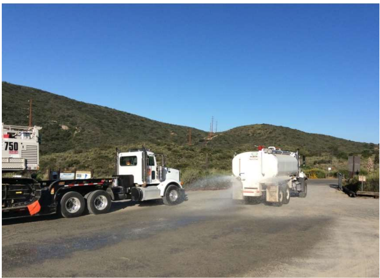
Photo 1: In accordance with APM AIR-02, water was applied to the unpaved access at the Sweetwater Staging Area (TL 625B) prior to crane demobilization.
