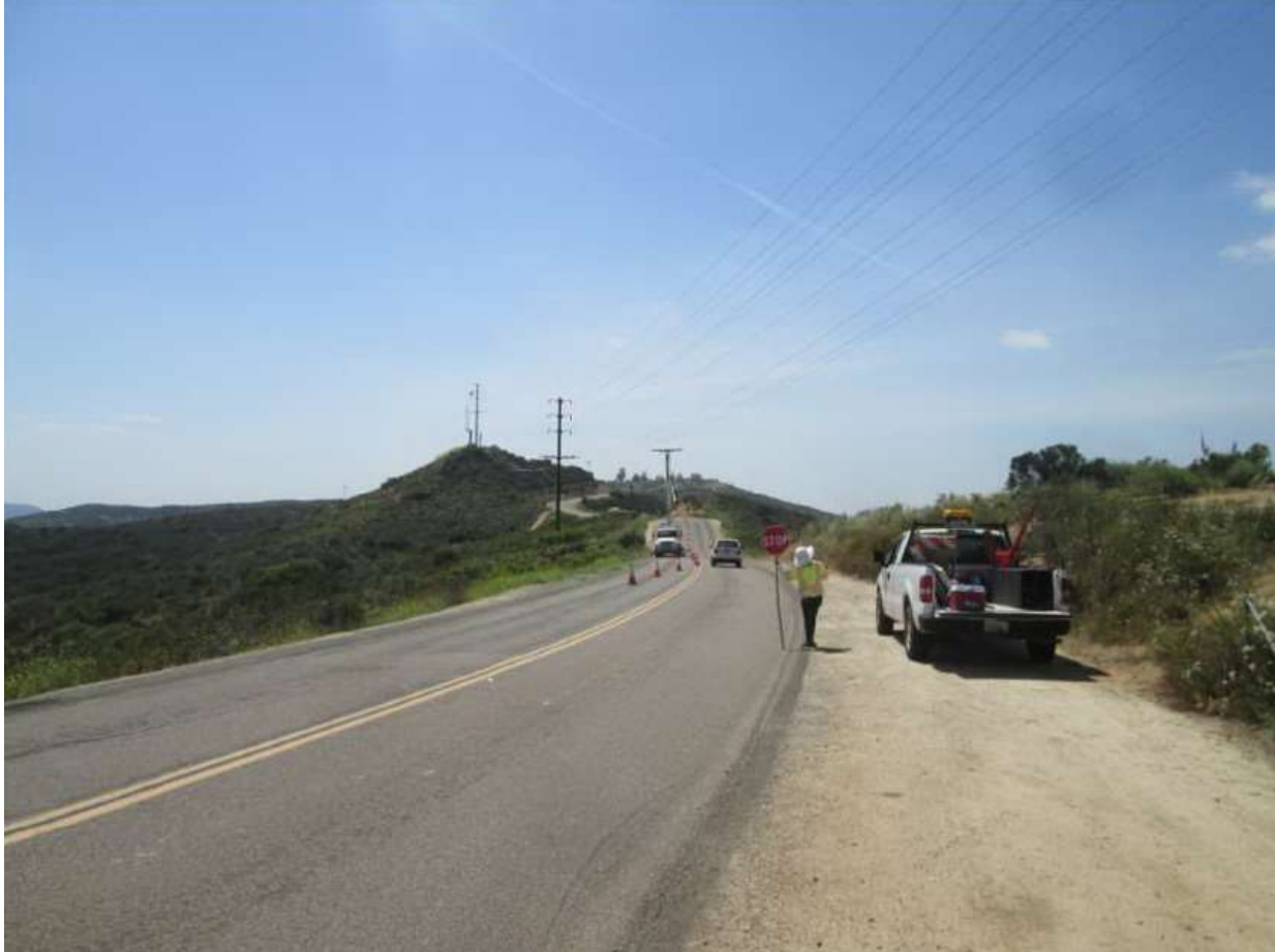
Photo 3: During placement of guard structures between Z272846 to Z272847 (TL 625B), traffic control was staged along Sequan Truck Trail in accordance with APM TRANS-02 and APM TRANS-05.
