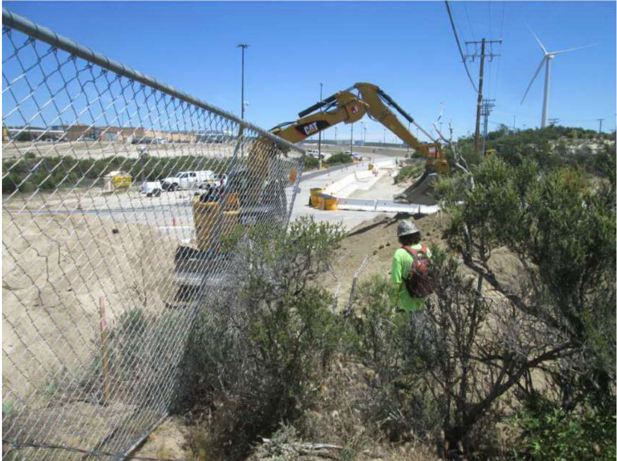
Photo 6: During excavation for the underground utilities along TL 629E, Native American monitors were noted observing activities in accordance with MM CUL-1.
