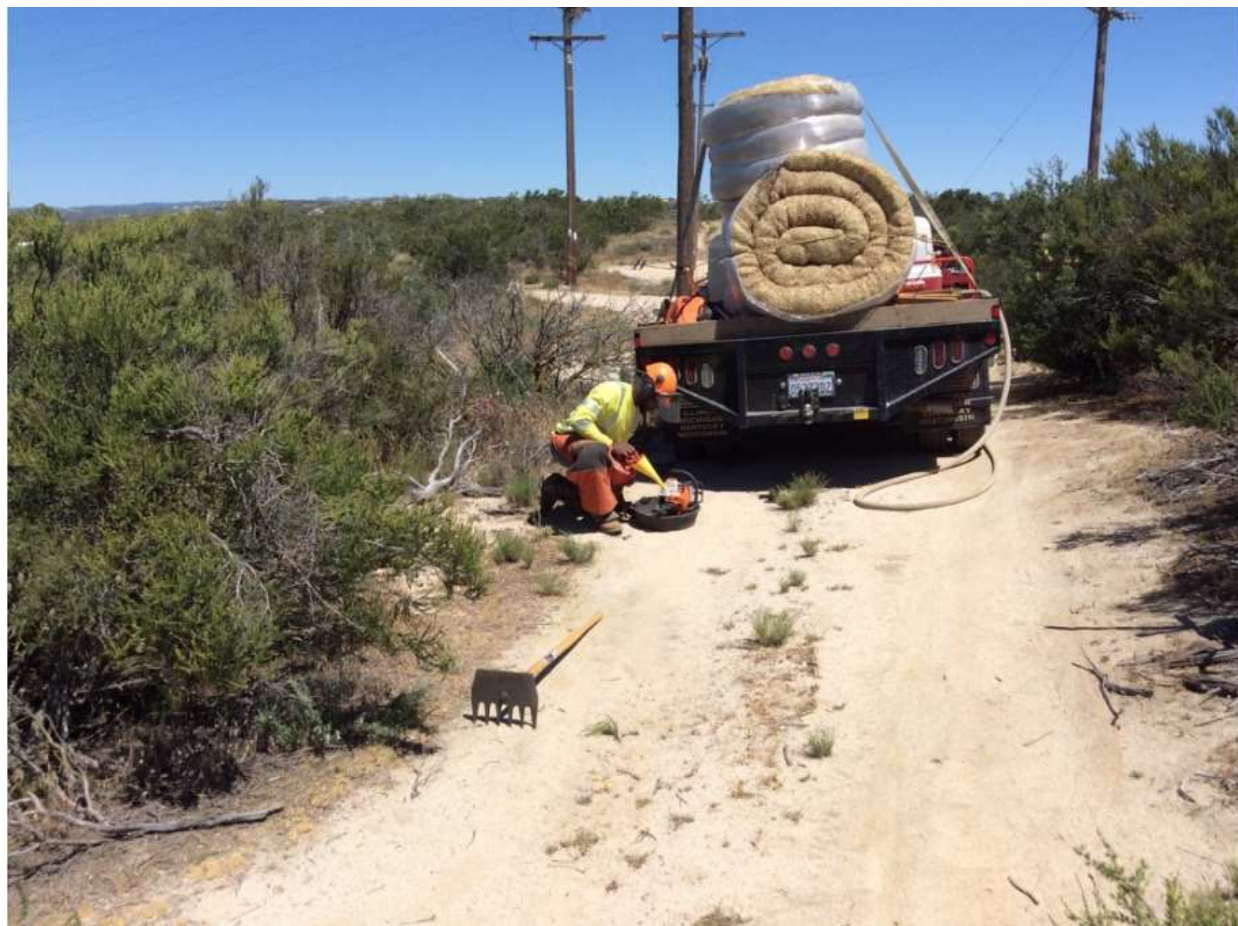
Photo 5: Crews were observed removing and chipping vegetation at Stringing Sites 16 & 17 near Pole Z44268 (TL 6931). In accordance with MM PHS-2, a drip pan was used during chainsaw fueling at Stringing Site 16.
